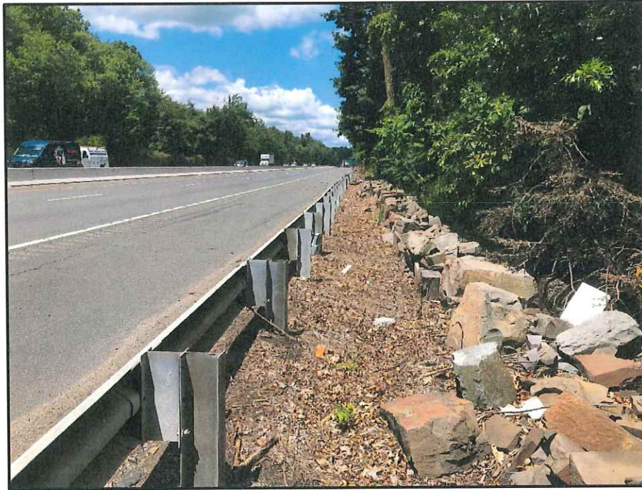
Photograph 3: View to the northwest of a rock wall adjacent to Route 208 NB
