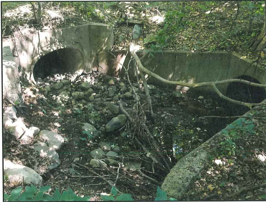
Photograph 11: View to the north of the proposed culvert replacement adjacent to Route 208 SB
