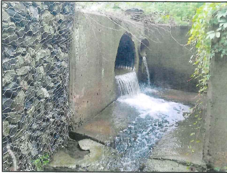
Photograph 1: View to the northwest of culvert and gabion wall adjacent to James Way and Route 208 NB
