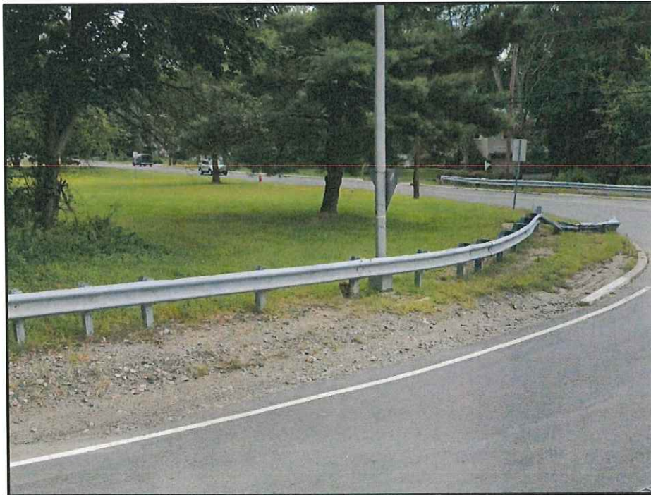
Photograph 8: View to the west of proposed guiderail replacement along on-ramp for Route 208 NB
